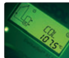
Illuminated system-monitoring display
